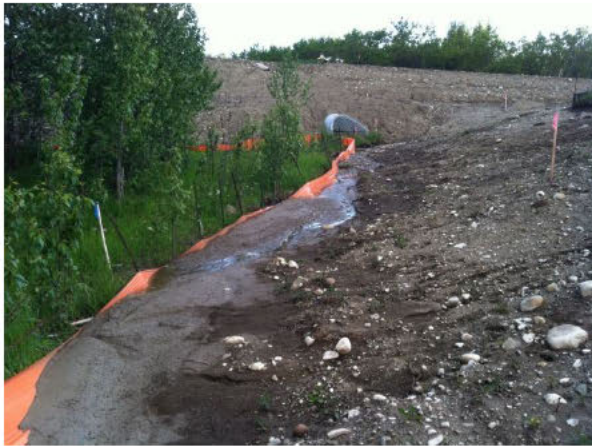
Figure 2. Photo taken on June 18 2013 , showing a drain installed by Silverhorn that channels storm water flow directly towards Equestrian Estate. This photo also highlights the level of erosion created by Silverhorn when they removed an extensive amount of trees and vegetation.
