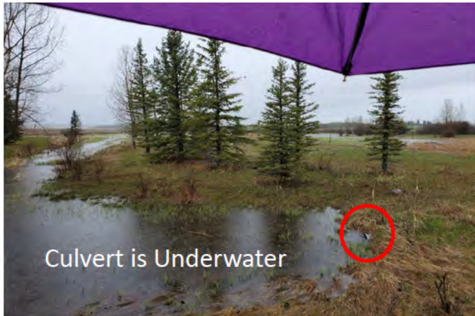
Swale is Inundated
