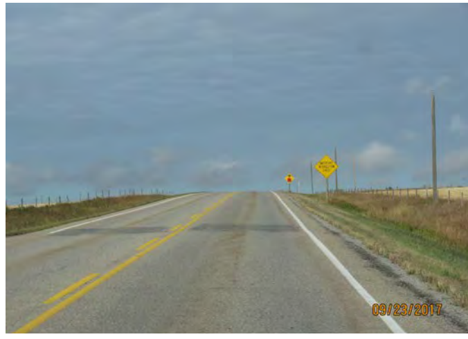
Photo 10: approaching intersection with poor intersection sight distance.
